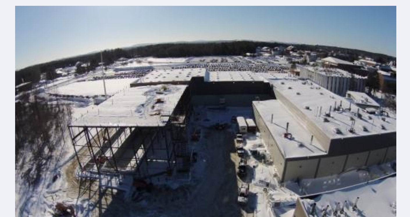
Aerial photograph taken on February 15, 2015 showing the wind wave laboratory under construction
