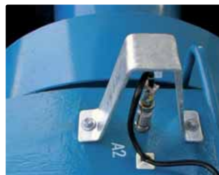
CMS sensor for the low-speed shaft of the gearbox
